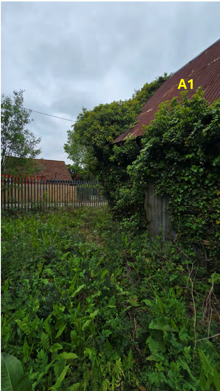
Figure 11. Former access between the Traditional Sussex Barn (A1) and B1. Subject of the milk tanker accident during the 1980s.
