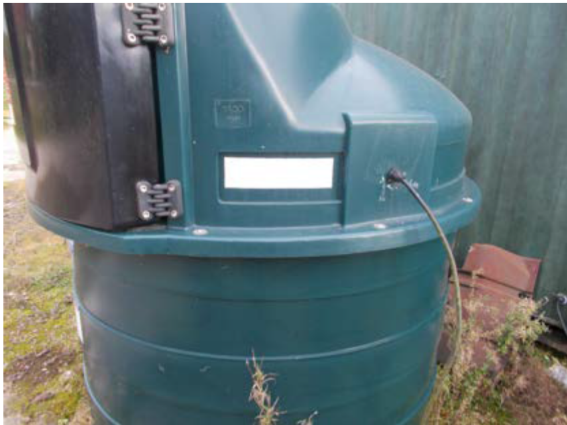
Diesel fuel storage tank
