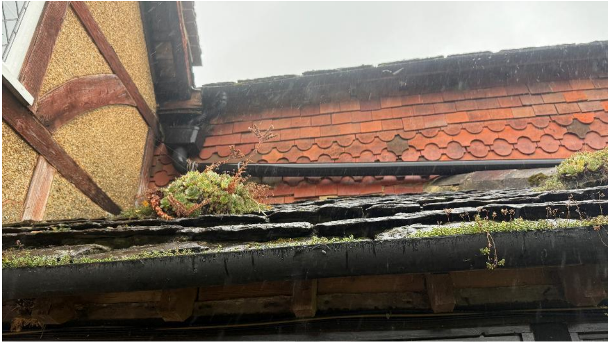
External note 2 – gaps at eaves, beneath hanging tiles and roof stone tiles
