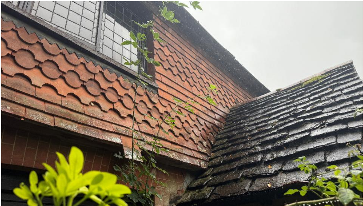
External note 6 - gaps at eaves, beneath hanging tiles and roof stone tiles
