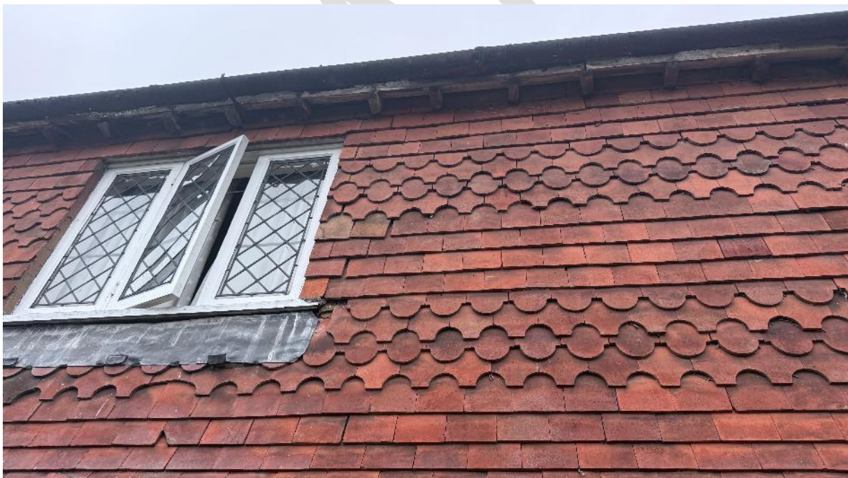
External note 1 – gaps at eaves, beneath hanging tiles and flashing detail
