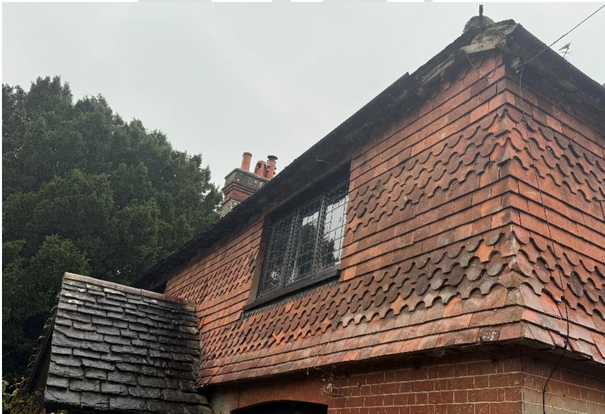
External note 5 - gaps at eaves, beneath hanging tiles and roof stone tiles
