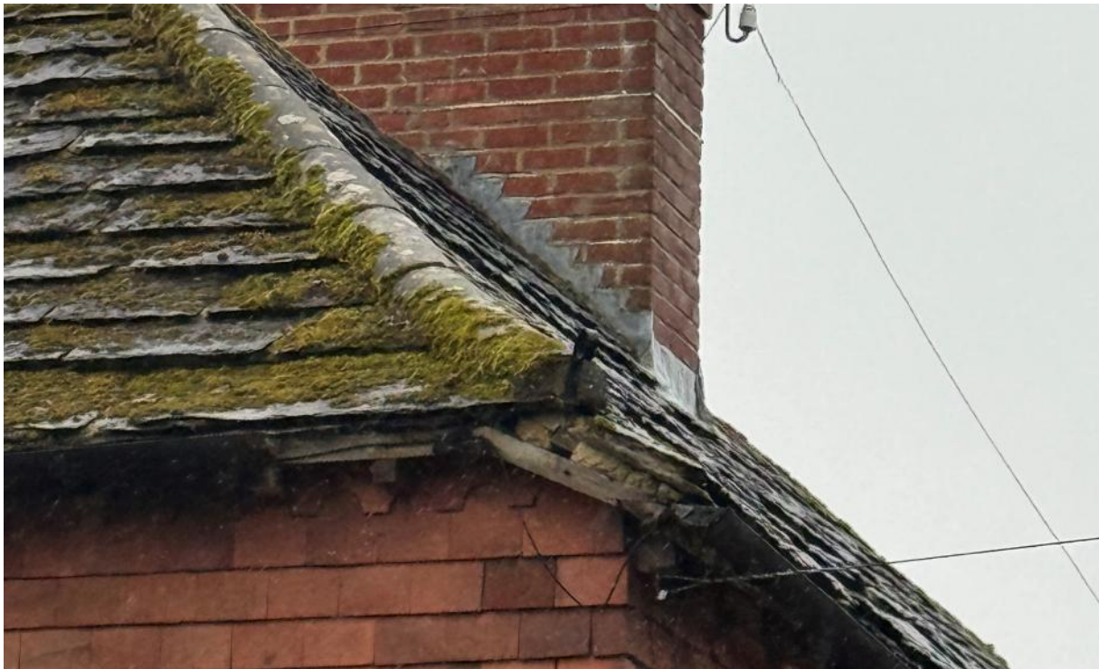
External note 4 – Missing gutter leading to heavily water damaged corner, gaps beneath hanging tiles and roof stone tiles
