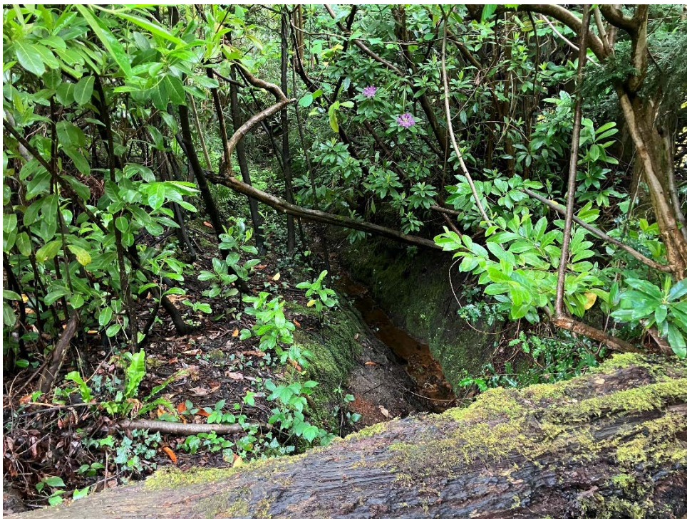
Photograph 52: Drainage infrastructure in northwestern area of site.
