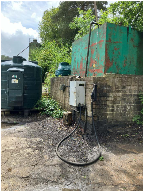
Photograph 36: Fuel storage area with pump. Looking south.
