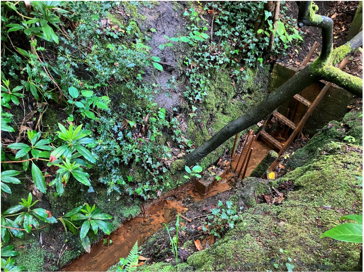
Photograph 51: Drainage infrastructure in northwestern area of site.
