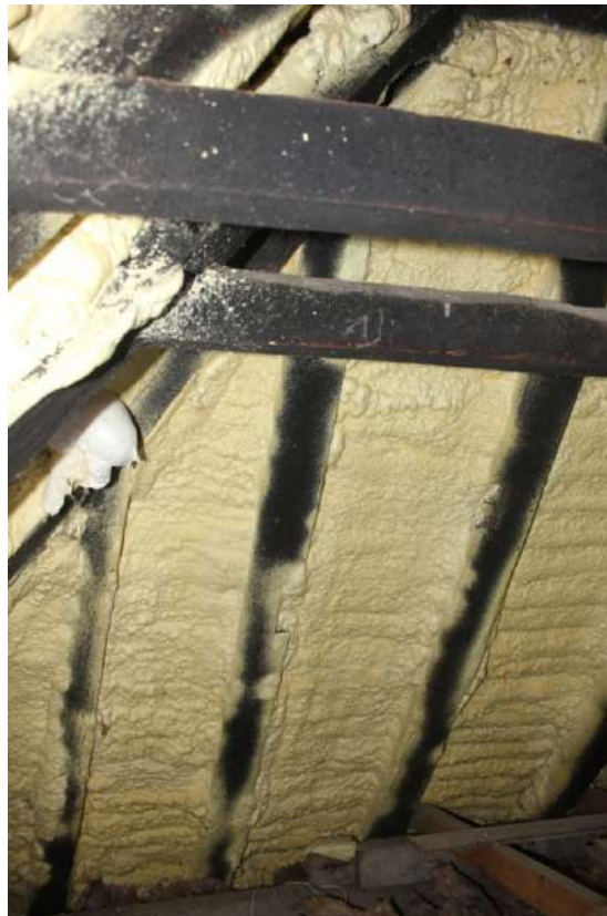
Plate 14. Heavily sooted roof space in Bay 1.
