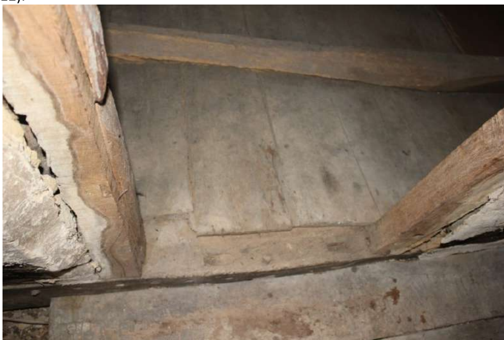
Plate 18. The tiebeam in Truss C with lack of soot staining in the middle, which is heavily stained towards the outer edges of the beam.
