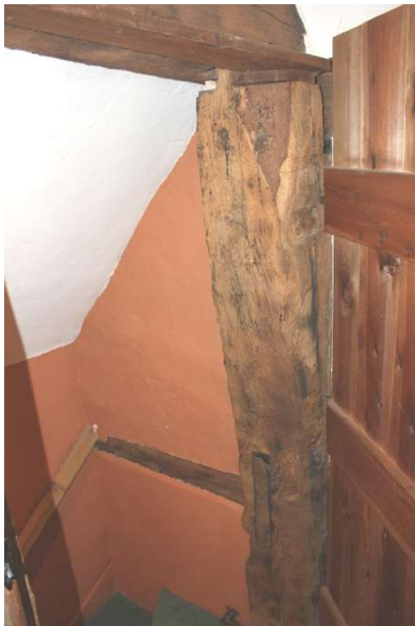
Plate 63. Cut head brace in the south-west corner of Truss A.
