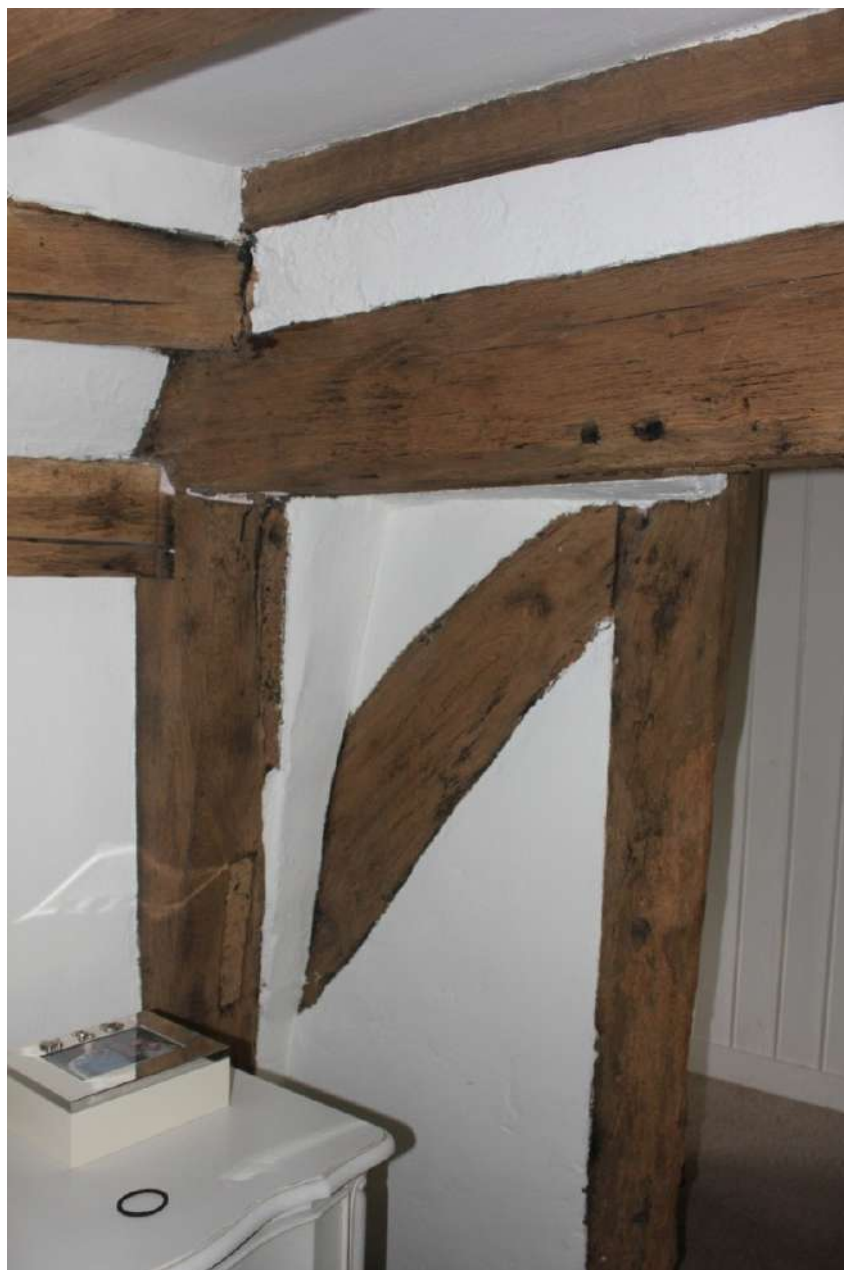
Plate 7. No principal rafters jointed into the tiebeam of Truss D.
