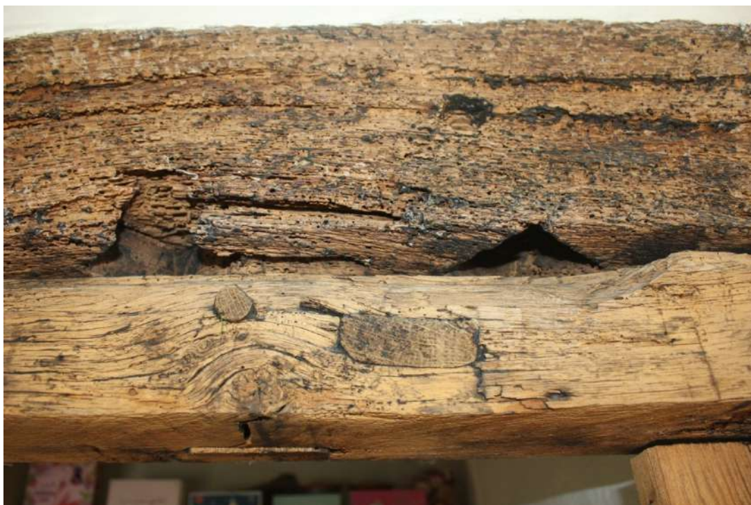
Plate 10. Empty diamond shaped mullions in the soffit of the side girt in the far south side of Bay 2.
