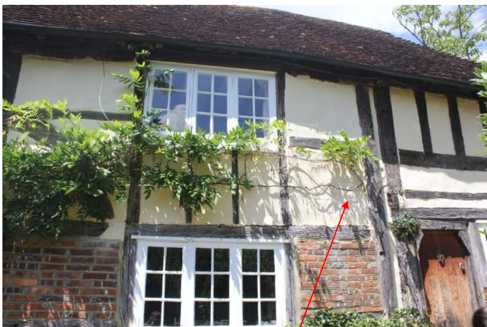
Plate 6. Missing foot brace next to the location of the former hall window.
