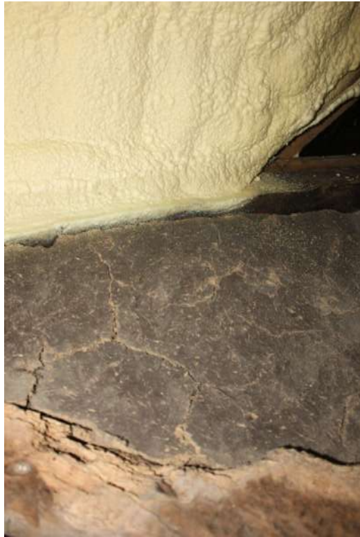
Plate 33. Soot staining in the north side of the panel which separates the two ranges.
