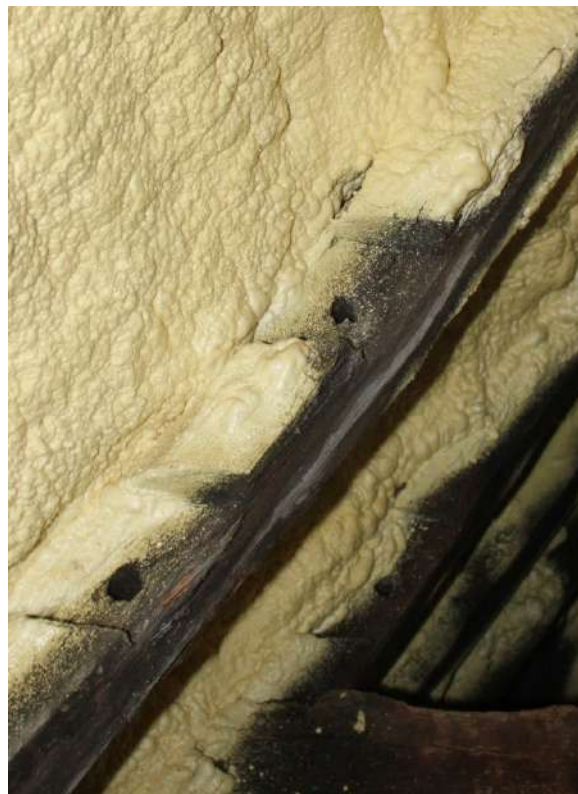
Plate 15. Two phases of missing collars in the Bay 1 roof, both equally sooted.
