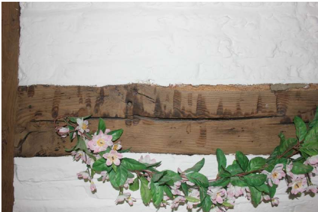
Plate 50. Significant taper marks on the first floor bressumer.
