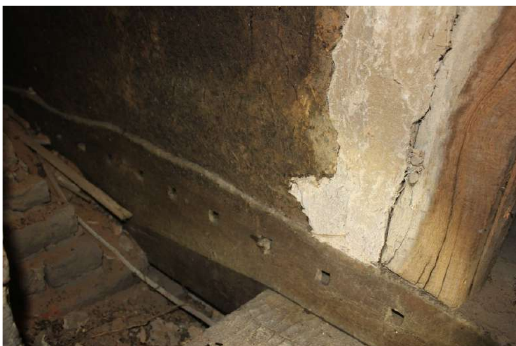
Plate 19. Square holes to the south side of the tiebeam.
