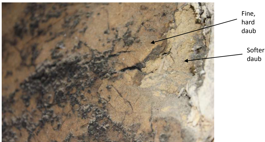
Plate 23. Two distinct layers of daub seen in section with the harder form on the face.
