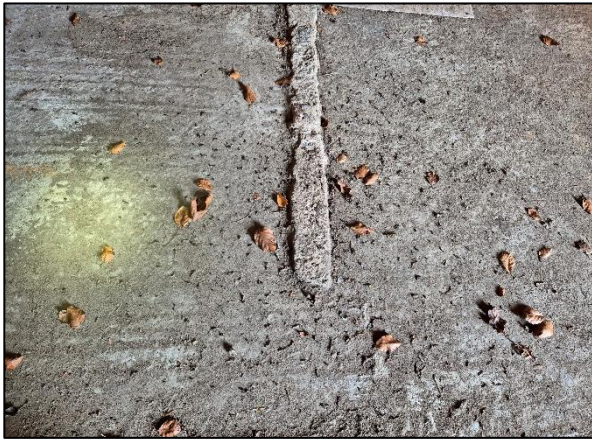
Photo 13: Barn 1 bat droppings found internally.
