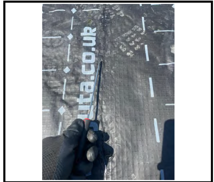
A mechanical point stress test being conducted upon a welded lap joint.
