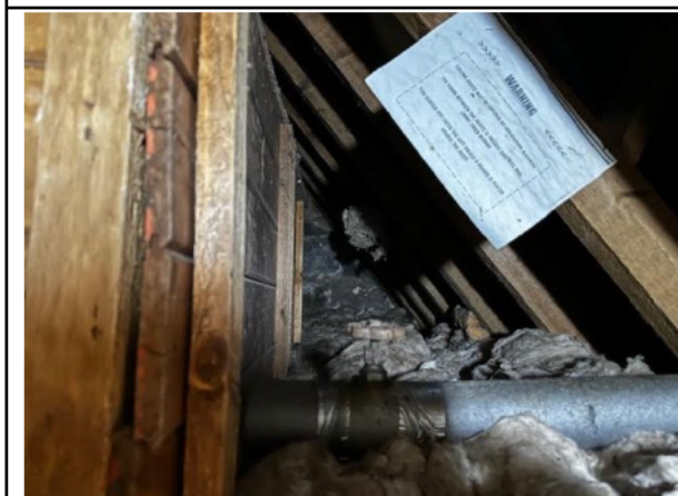
Photograph 11 – The void had very limited access in places. A sign in the void advised it was unsafe to enter and stated 'the floor between the joists was fragile and will not carry your weight. You should not enter the loft unless a board is placed across the joists'.
