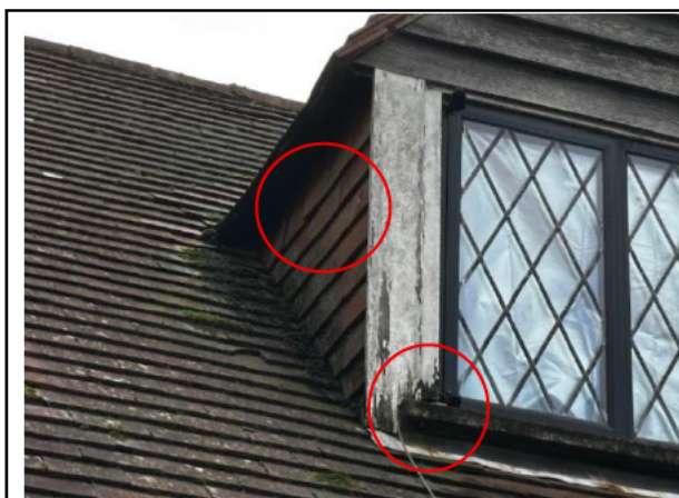
Photograph 7 – There was a lifted hanging tile on the side of the dormer window on the southeast elevation and gaps at the base of the rotten wooden window surround offering potential roost features (PRF's) for crevice-dwelling bats.
