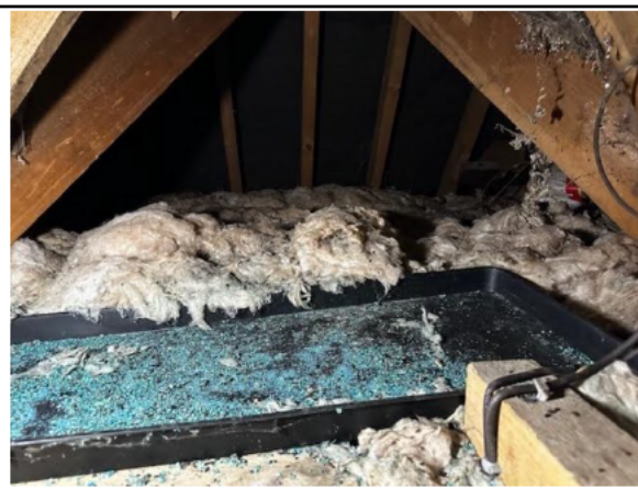
Photograph 10 – The main void in the dwelling was covered in bat and mouse droppings. There was also a lot of rodent poisoning across the void.
