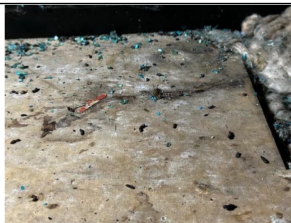
Photograph 12 – In addition to the mice droppings found, evidence in the form of bat droppings morphologically consistent with those of the brown long-eared species of bat was found scattered across the void.
