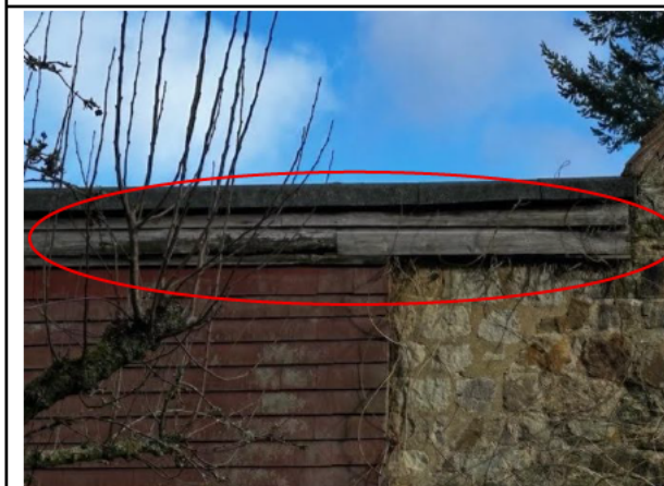
Photograph 9 – There were gaps under the wooden soffits and the edge of the flat roof on the southwest elevation presenting PRF's for bats.
