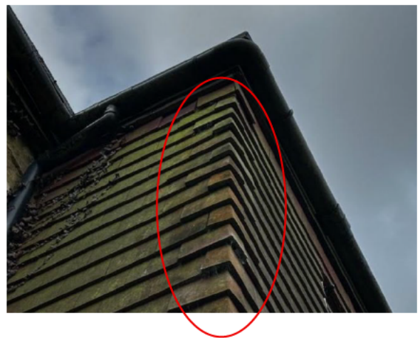
Photograph 6 – There were gaps under some of the hanging tiles along the edges, offering potential roost features (PRF's) for crevice-dwelling bats.
