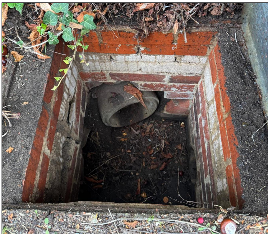
Figure 2.3 – Incoming Surface Water Pipe from Woodfalls to Manhole on Site Boundary
