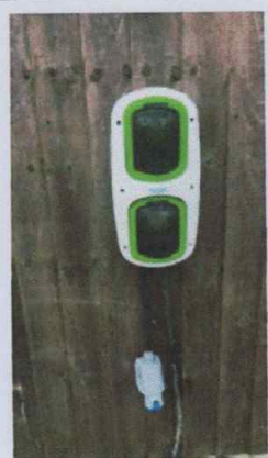
Electric vehicle charging point
