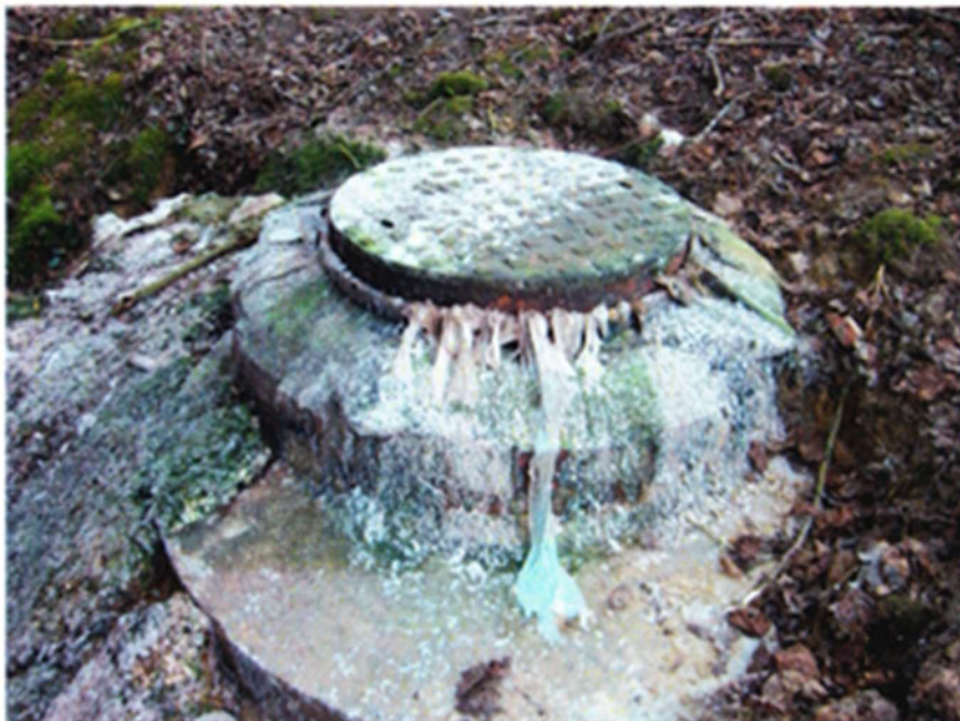
Close-Up of the Manhole with Raw Unscreened and Untreated Sewage Overflowing and Running Down the Bank and into Parsons Brook
