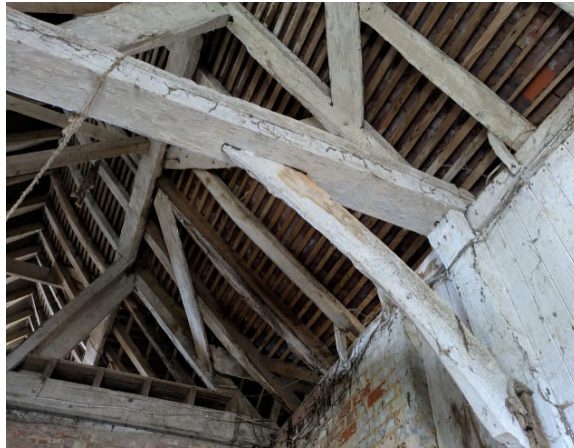
Photo 13: Internal view of northern section of B12 (with bat droppings below this mortise and tenon joint – see Photo 14).
