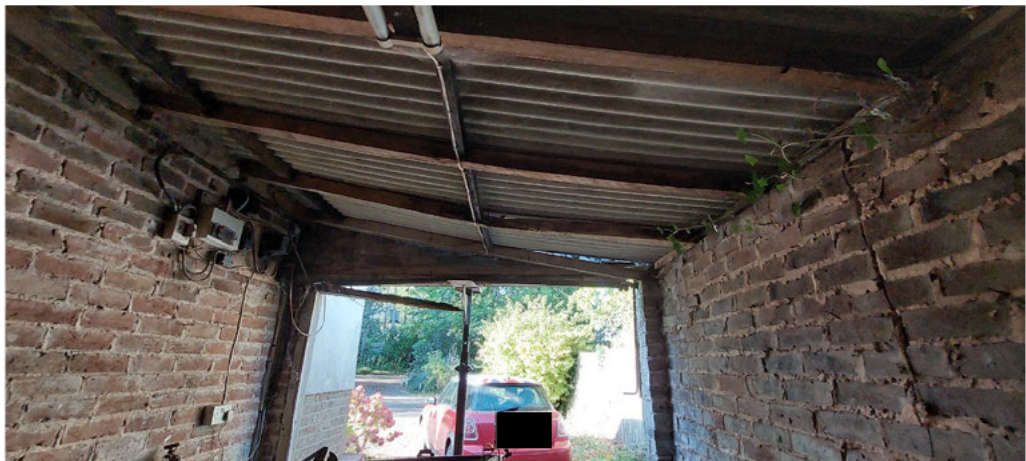
Photograph No: 8 – Internal view of B03 showing gaps in roofing. Open fronted aspect is likely to deter bat use.
