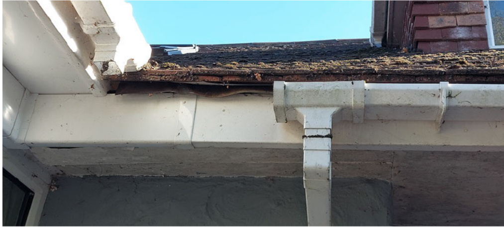
Photograph No: 6 – View of B01 roof and gaps in tiles and around soffits, creating roosting opportunities for crevice dwelling bat species.
