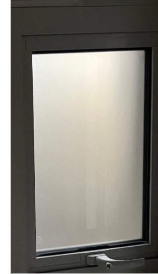
Condition 11: Obscured top hung Windows
