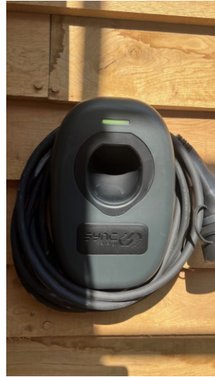
Condition 8: EV car charger
