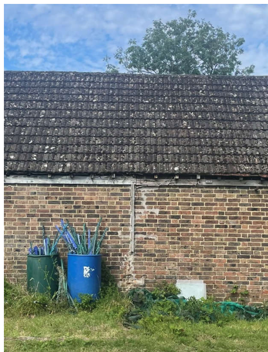
Cracking at centre of East elevation
