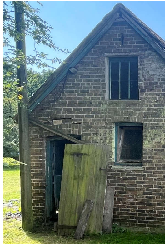
Failed soldier arch over door in North elevation
