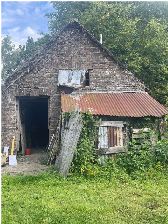
Failed soldier arch over door in South elevation. See a narrow soldier courses as evidence of earlier window
