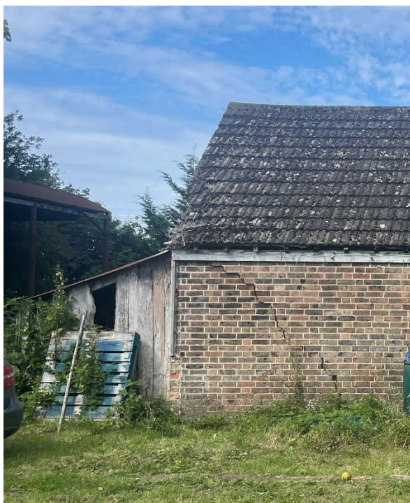
Cracking to southern end of East elevation
