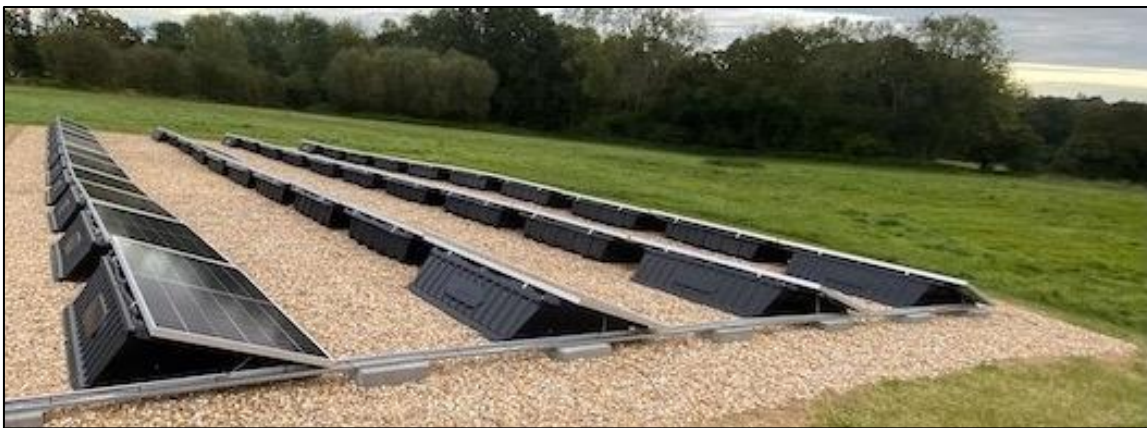
Example of the installer's ground mounted solar panel set up
