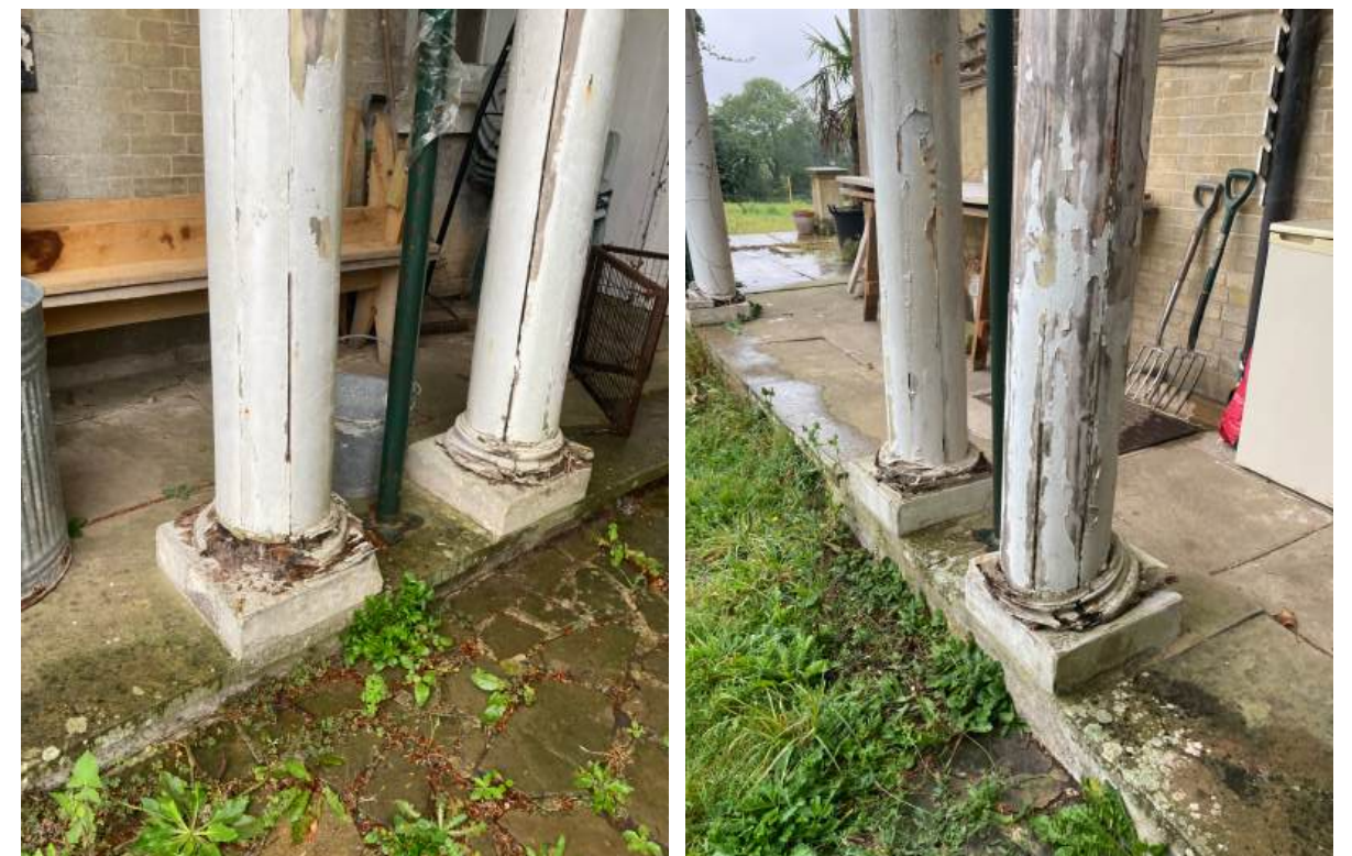
Details showing the poor condition of the veranda
