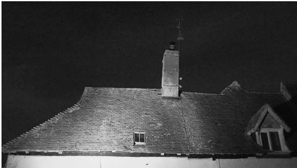
Fig. 15 – IR camera view of the house, from W
