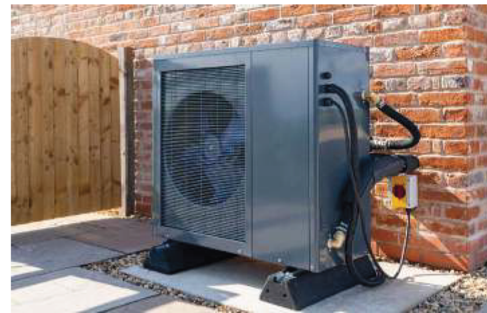
Air Source Heat Pump
