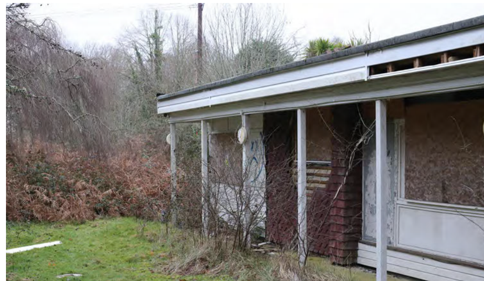
Site Photograph D. Poor state of repair of built form on Site.
