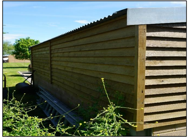
Photo 6: Tight weatherboarding and roof joins.
