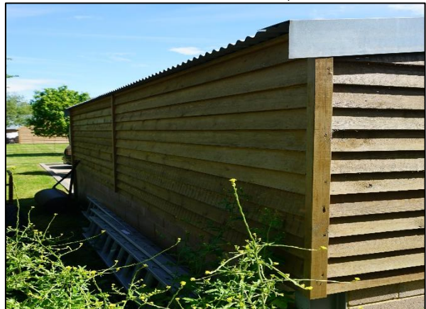
Photo 6: Tight weatherboarding and roof joins – northern boundary.
