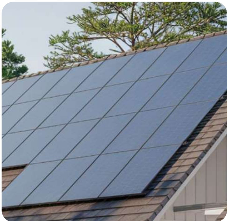
New photovoltaic panels will provide the building with a renewable source of electricity reducing reliance on the national grid.
