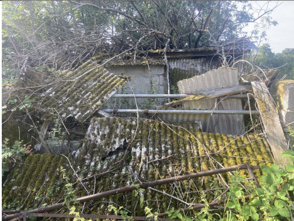
Photo 7: Asbestos roofing noted onsite
