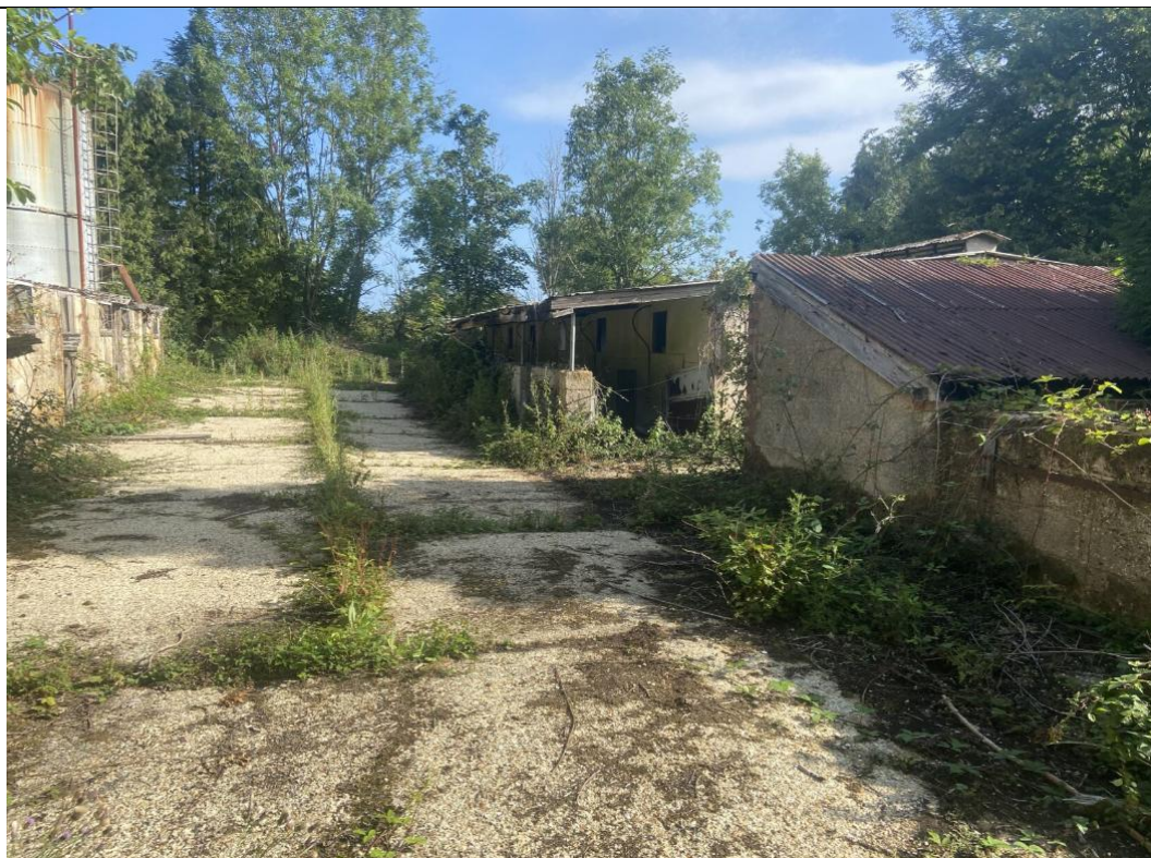
Photo 3: asbestos roofing materials noted
