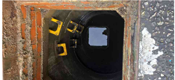
MH22X_36af7140-474c-43e1-a1e5-436e68e3ebf7_20241125_100827.jpg, 00:00:03, 0.00 m General remark, LINE HOLDING, MH24 REQUIRES EMPTYING
