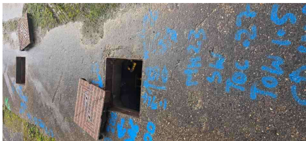
MH23X_7e7af6c9-528c-478b-9e05-63c4d5869097_20241125_100835.jpg, 00:00:03, 0.00 m General remark, INTERCEPTOR MH24 REQUIRES EMPTYING TO SURVEY
