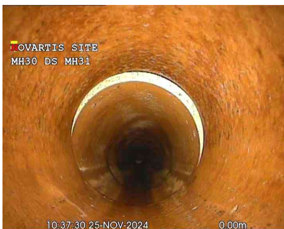
MH30X_be1fa4e2-0bad-4938-8c7d-66491d64b79e_20241125_104944_019.jpg, 00:00:10, 0.28 m Joint displaced, large
