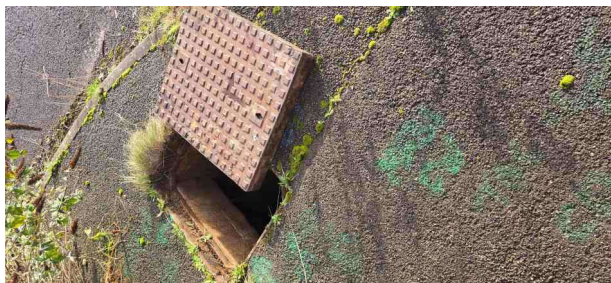
MH31X_1b539d62-dc46-4c8c-884b-19607f4dc15a_20241125_104636.jpg, 00:00:01, 0.00 m Start node, manhole, reference: MH31
