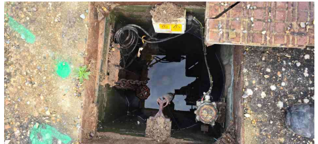
MH32X_6476d4ac-80fb-4081-a5f3-cf29dca6fb3d_20241125_112757.jpg, 00:00:55, 14.78 m Finish node, manhole, reference: MH32, PUMP IN CHAMBER, NOT WORKING
