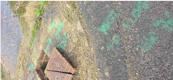
MH32X_7bcfddd9-202f-4e2b-82db-48c6380e95e6_20241125_112750.jpg, 00:00:55, 14.78 m Finish node, manhole, reference: MH32, PUMP IN CHAMBER, NOT WORKING
