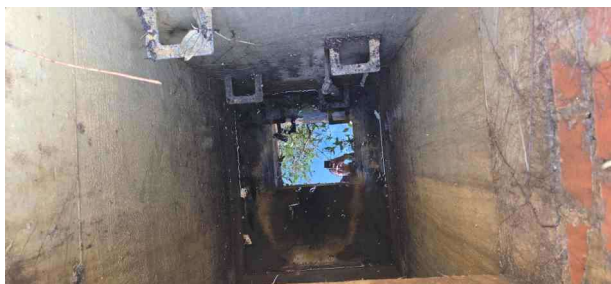
MH27X_752d7050-5c7c-4b6d-8922-7f7d2ea637d2_20241125_113301.jpg, 00:00:03, 0.00 m General remark, REQUIRES SUCKING OUT TO SURVEY
