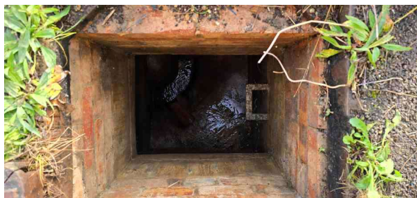
MH31X_a5845c64-2fc7-405d-9f44-63ba8d392b8f_20241125_104917.jpg, 00:01:07, 14.10 m Finish node, manhole, reference: MH41
