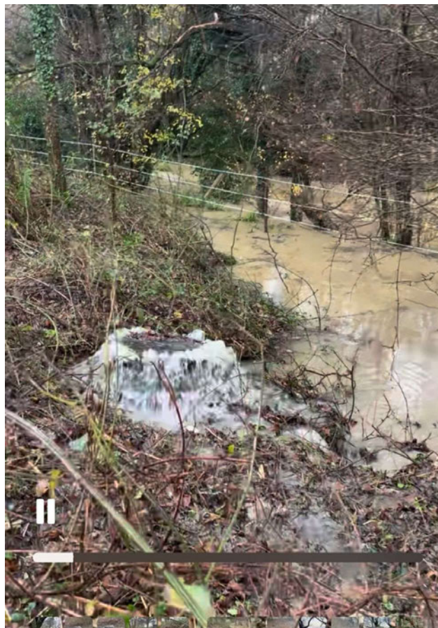
Still from a Video of the Same Manhole on Another Occasion
