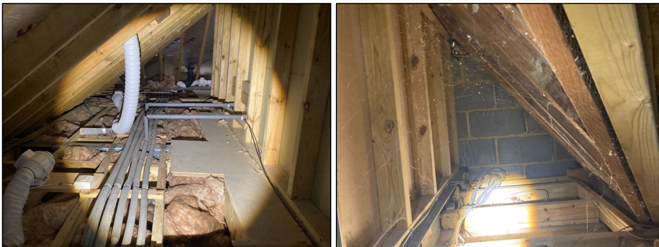
Photograph 1a & 1b. A view of the largest section of Void 1 (left), with a smaller “lip” section present at the end of the void.
