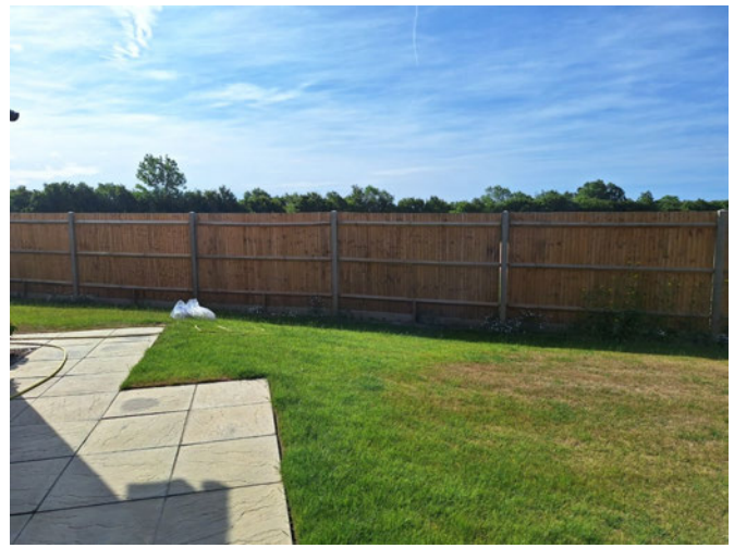
Plate 2: The asbestos fibres were found adjacent to a newly installed fence post.
