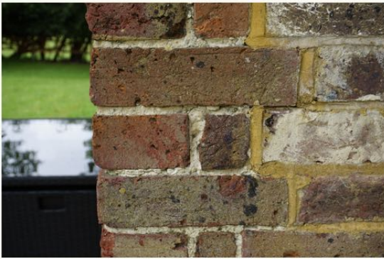
DATED ERODED BRICKWORK
