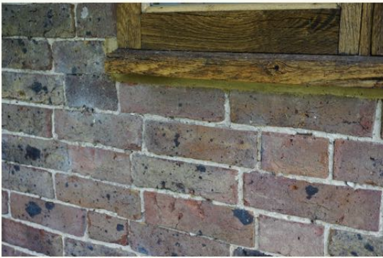
WEATHER DATED BRICKWORK
