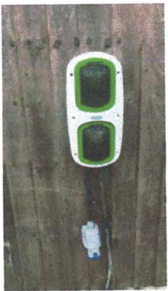
Electric vehicle charging point
