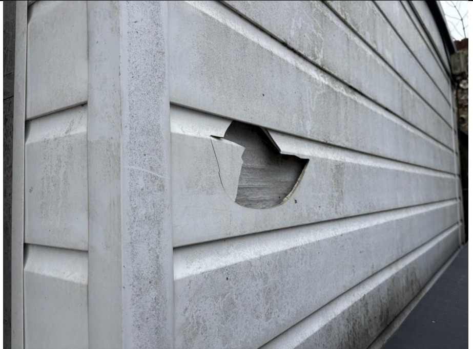
Photograph 5: Hole in PVC facing on western aspect
