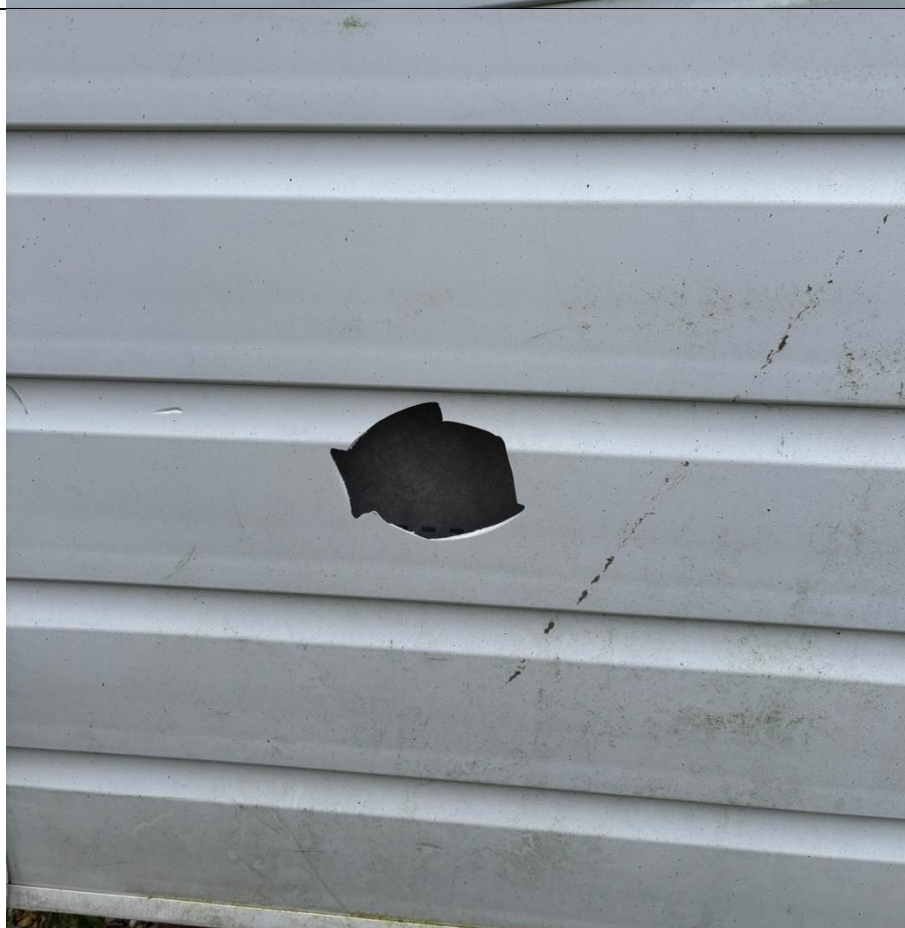
Photograph 4: Hole in PVC facing on northern aspect
