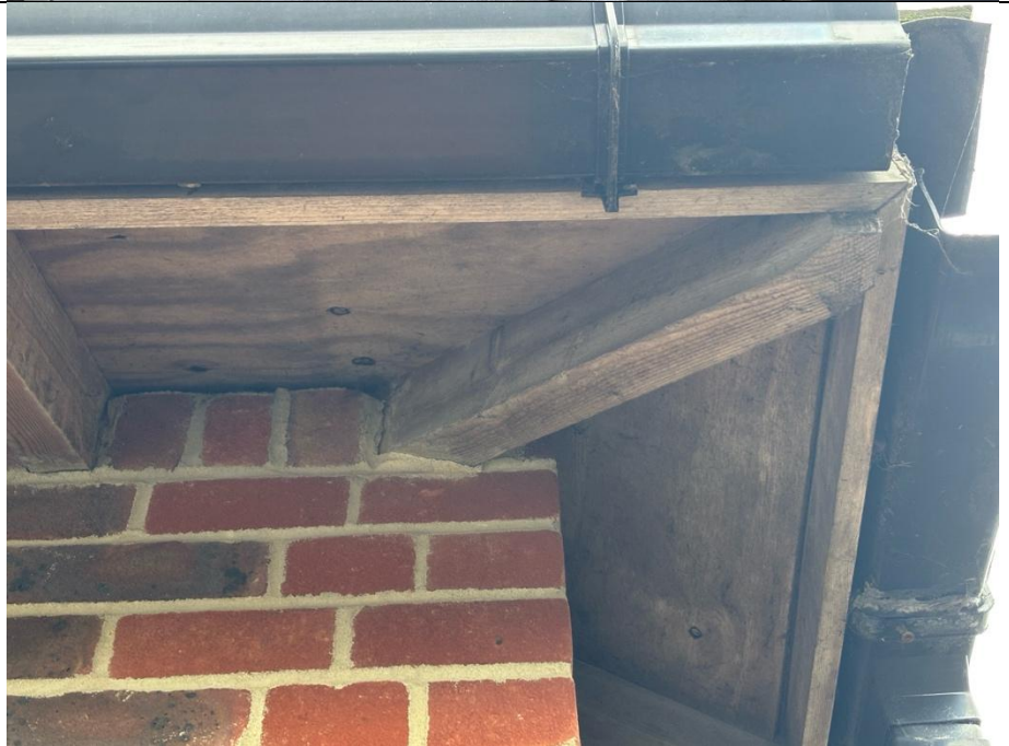
Photograph 6: Changing room wooden soffit and gap providing potential access for bats into the loft void
