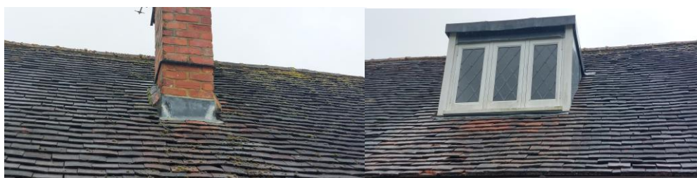
Photographs 01 and 02 – Gaps around flashing along eastern elevation and gaps between tiles / missing tiles along western elevation.
