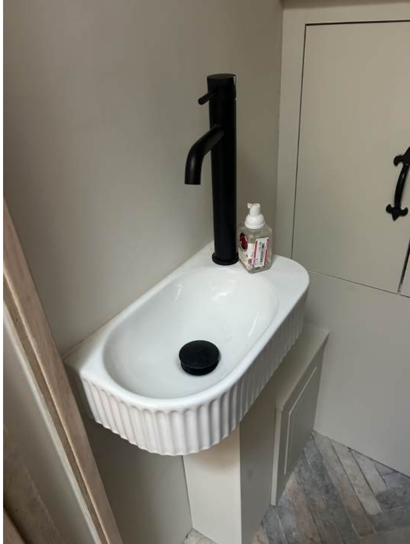
Utility Sink Mixer Tap – Photo 3 Assumed flow rate: 6.0 l/min
