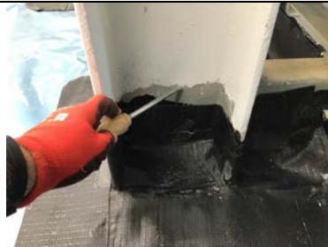
Probe testing a steel stanchion detail in unit 1.
