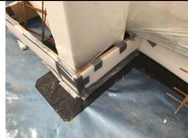
Steel stanchion covered with miothene at the time of our inspection.
