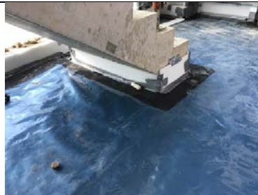
Miothene was placed around the base of the stairs at the time of our inspection.
