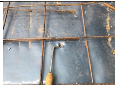
Damage found in the membrane at the time of our inspection.
