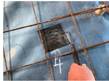
4. Defect was patched repaired by during inspection using Juta GP1 SAM and probe tested.
