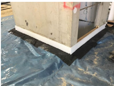
The lift pit detailing had been covered with miothene at the time of our inspection.
