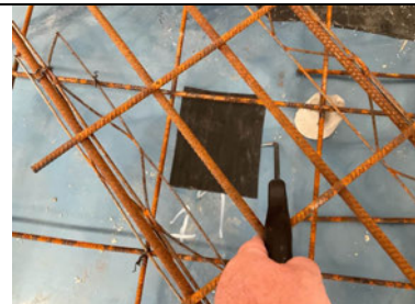
1. Defect was patched repaired by during inspection using Juta GP1 SAM and probe tested.
