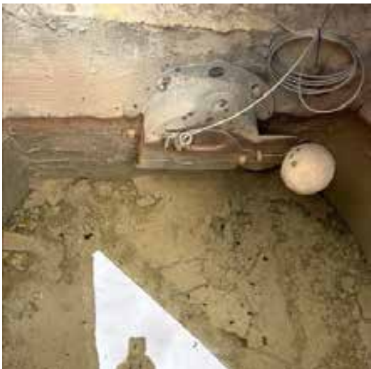
Existing carpark hydrobrake, IC 1 – May 2026
