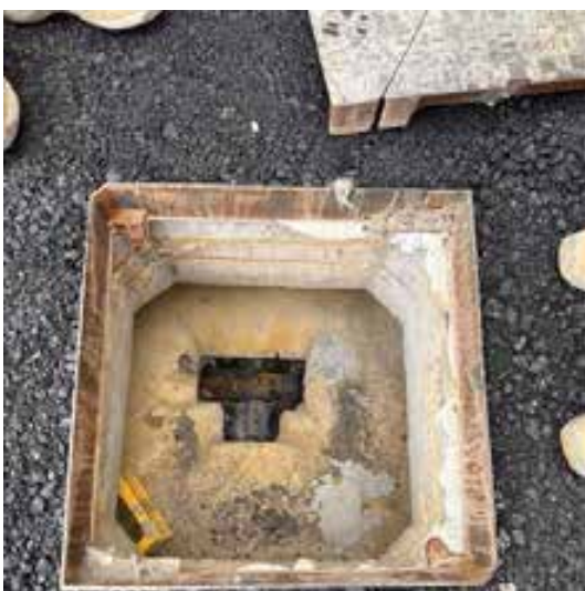
Existing surface water collection manhole (from Unit 12) – IC.2 – May 2026
