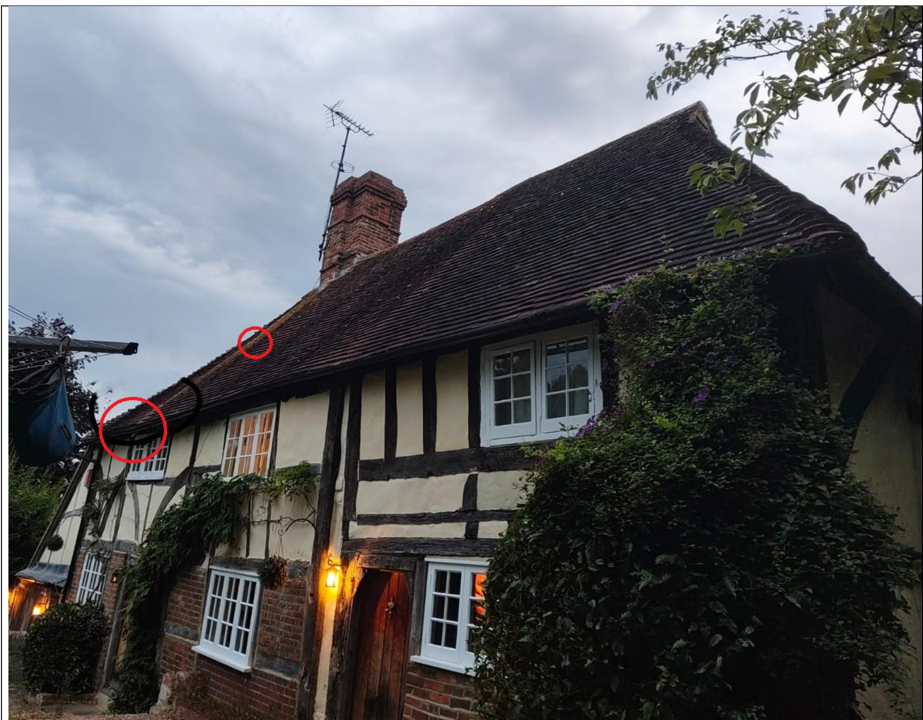
Figure B1 South-eastern side of the roof with 1x open soffit emergence and a roof tile emergence above.
