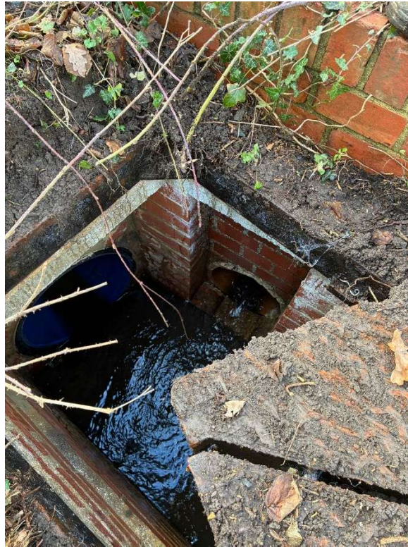
Image 17: 300mm diameter outfall from Sports Centre / School with 450mm diameter onward pipe
