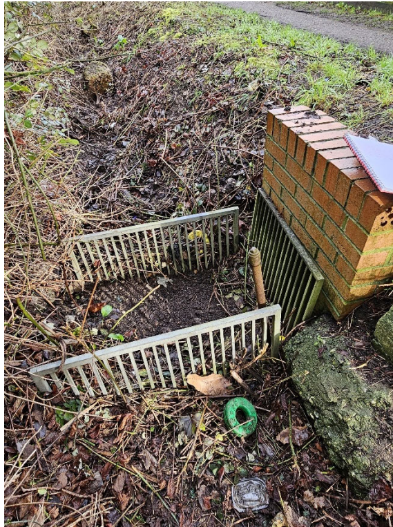
Image 08: Outfall from rear of houses on Shooting Field
