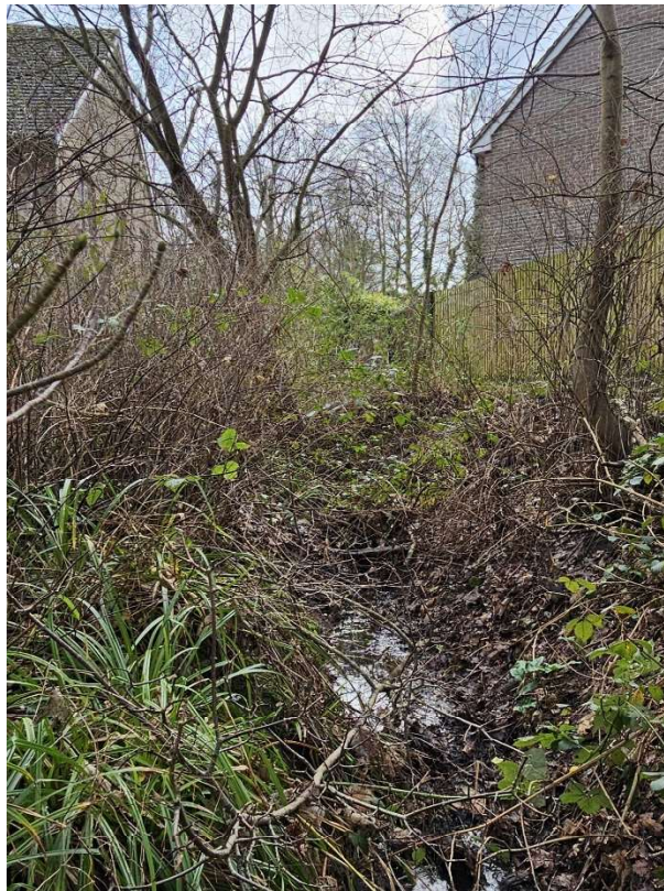
Image 24: Ditch to the south of Reads Walk, looking south. Too overgrown to approach the culvert below Reads Walk
