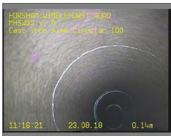
Photo: 33_33_190_A.JPG 0.16m, Crack, circumferential, from 12 to 12 o'clock
