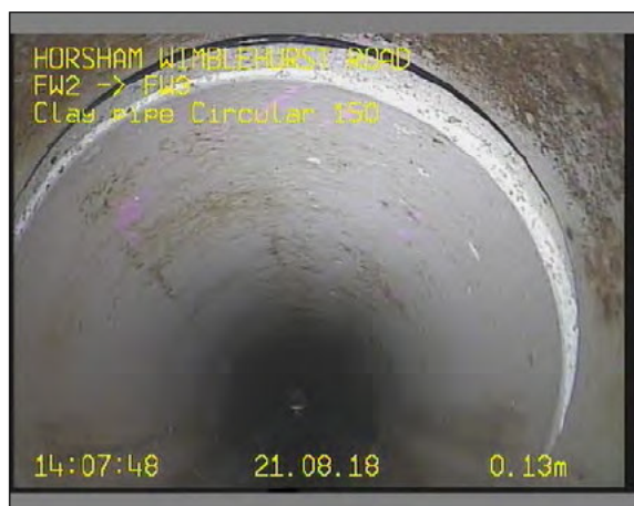
Photo: 12_12_53_A.JPG 0.13m, Joint displaced, medium
