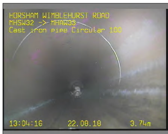
Photo: 21_21_118_A.JPG 3.76m, Crack, circumferential, from 12 to 12 o'clock
