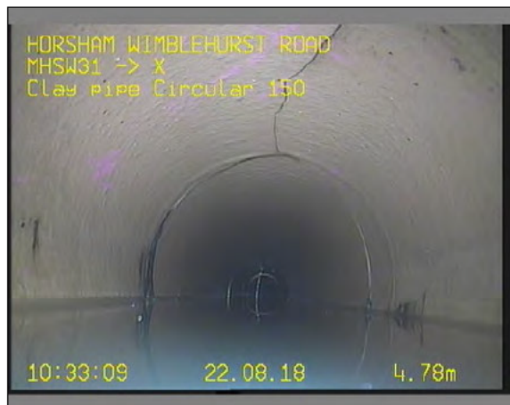
Photo: 16_16_84_A.JPG 4.76m, Fracture, longitudinal, at 12 o'clock
