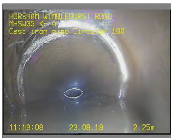
Photo: 33_33_194_A.JPG 2.25m, Broken pipe, from 12 to 12 o'clock
