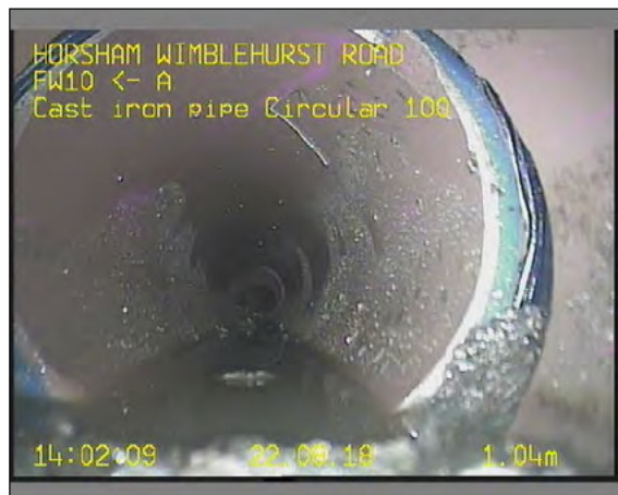
Photo: 22_22_124_A.JPG 1.04m, Open joint, medium
