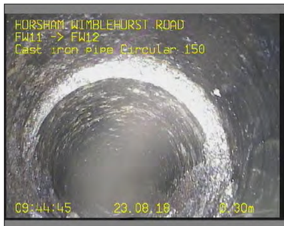
Photo: 31_31_179_A.JPG 0.3m, Joint displaced, medium
