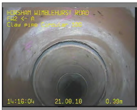
Photo: 13_13_60_A.JPG 0.39m, Crack, circumferential, from 6 to 12 o'clock
