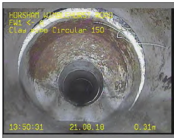
Photo: 9_9_35_A.JPG 0.31m, Joint displaced, medium
