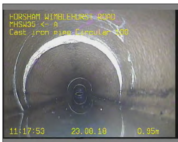
Photo: 33_33_192_A.JPG 0.95m, Crack, circumferential at joint, from 12 to 12 o'clock
