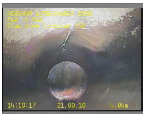
Photo: 12_12_55_A.JPG 4.84m, Crack, longitudinal, at 12 o'clock
