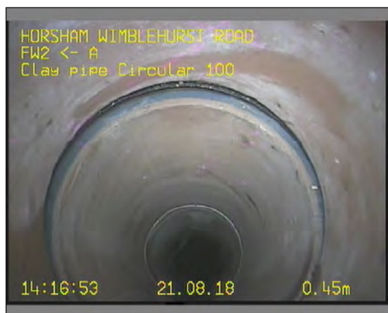
Photo: 13_13_61_A.JPG 0.45m, Joint displaced, medium
