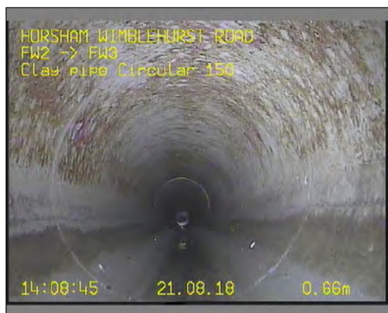
Photo: 12_12_54_A.JPG 0.66m, Crack, circumferential, from 12 to 12 o'clock
