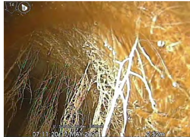
S 21X_3457e390-909a-4c8a-a44c-4650307ab933_20210518_1 55216_988.jpg, 00:01:37, 2.52 m Roots, mass, 25% % cross-sectional area loss
