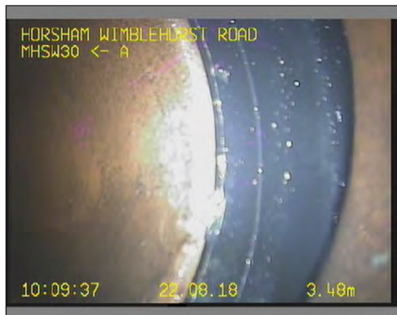
Photo: 14_14_70_A.JPG 3.48m, Joint displaced, medium
