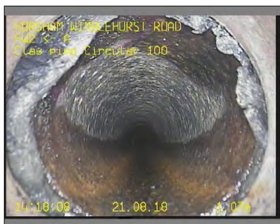
Photo: 13_13_62_A.JPG 1.07m, General remark Remarks: CONCRETE AROUND JOINT
