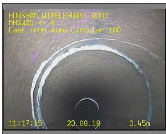
Photo: 33_33_191_A.JPG 0.45m, Fracture, circumferential at joint, from 6 to 3 o'clock
