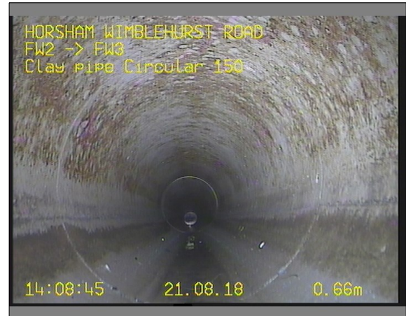
Photo: 12_12_54_A.JPG 0.66m, Crack, circumferential, from 12 to 12 o'clock
