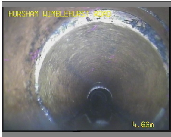
Photo: 29_29_167_A.JPG 4.66m, Fracture, circumferential, from 12 to 6 o'clock
