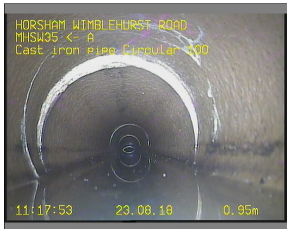
Photo: 33_33_192_A.JPG 0.95m, Crack, circumferential at joint, from 12 to 12 o'clock
