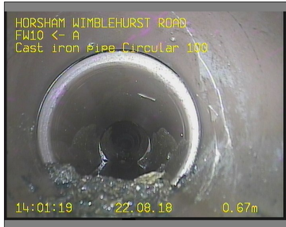
Photo: 22_22_122_A.JPG 0.67m, Crack, circumferential, from 12 to 5 o'clock
