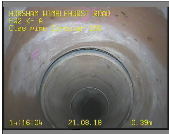
Photo: 13_13_60_A.JPG 0.39m, Crack, circumferential, from 6 to 12 o'clock
