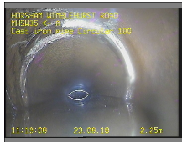
Photo: 33_33_194_A.JPG 2.25m, Broken pipe, from 12 to 12 o'clock
