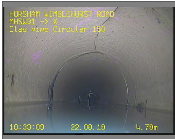
Photo: 16_16_84_A.JPG 4.76m, Fracture, longitudinal, at 12 o'clock
