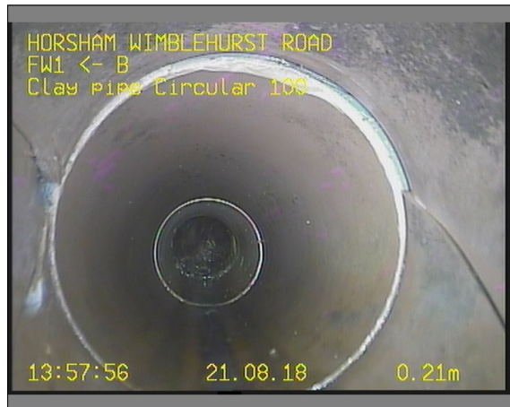
Photo: 10_10_45_A.JPG 0.21m, Fracture, longitudinal at joint, at 8 o'clock
