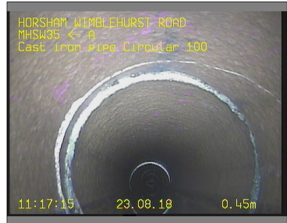
Photo: 33_33_191_A.JPG 0.45m, Fracture, circumferential at joint, from 6 to 3 o'clock
