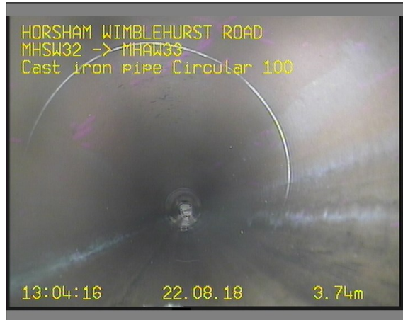
Photo: 21_21_118_A.JPG 3.76m, Crack, circumferential, from 12 to 12 o'clock
