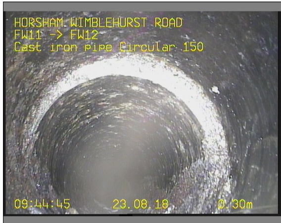
Photo: 31_31_179_A.JPG 0.3m, Joint displaced, medium
