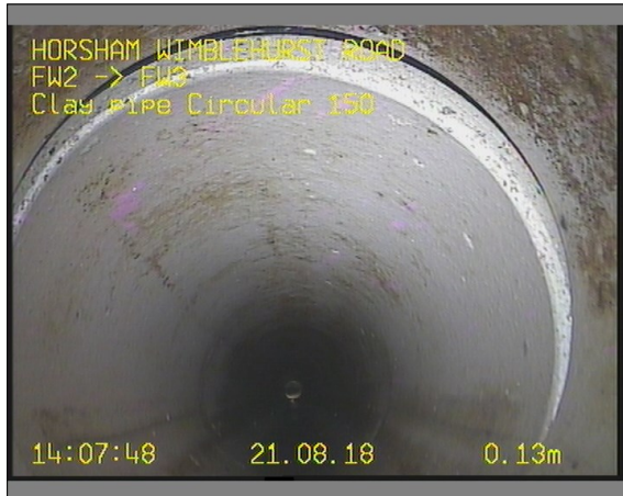
Photo: 12_12_53_A.JPG 0.13m, Joint displaced, medium
