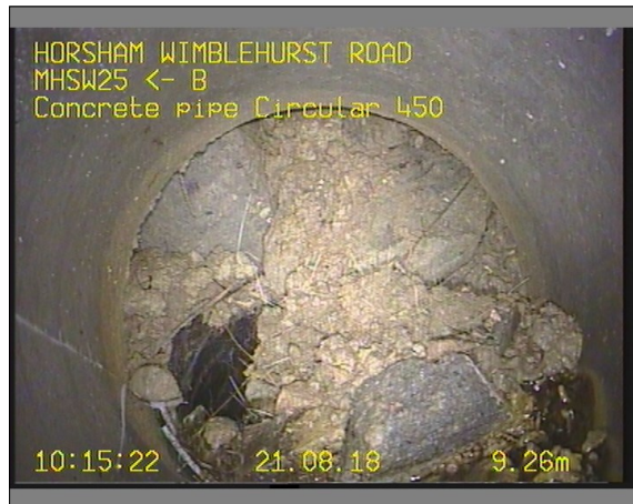
Photo: 3_3_9_A.JPG 9.26m, Survey abandoned Remarks: POSSIBLE COLLAPSE
