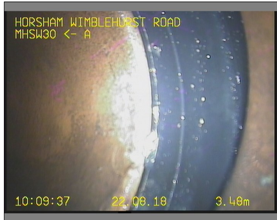
Photo: 14_14_70_A.JPG 3.48m, Joint displaced, medium
