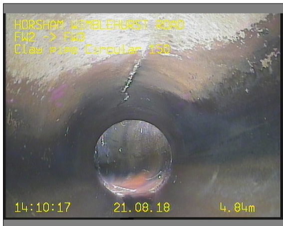
Photo: 12_12_55_A.JPG 4.84m, Crack, longitudinal, at 12 o'clock
