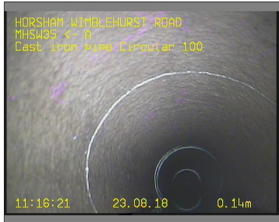
Photo: 33_33_190_A.JPG 0.16m, Crack, circumferential, from 12 to 12 o'clock
