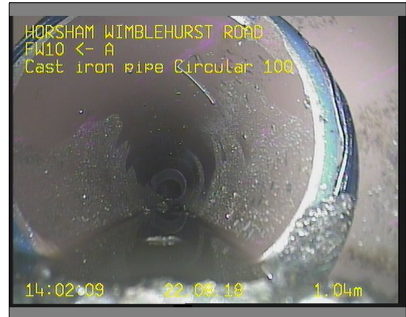
Photo: 22_22_124_A.JPG 1.04m, Open joint, medium
