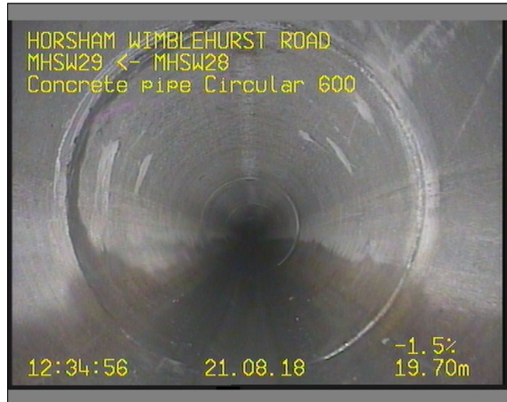
Photo: 7_7_27_A.JPG 19.7m, Infiltration, seeping at joint, from 6 to 12 o'clock
