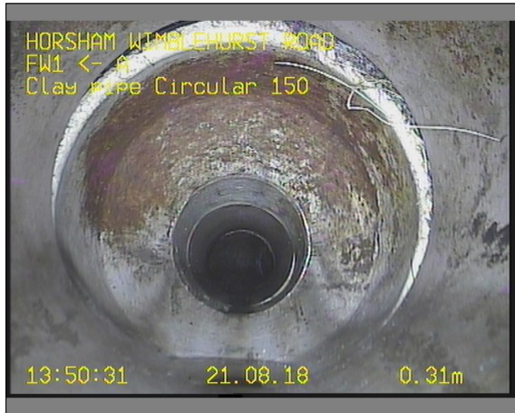
Photo: 9_9_35_A.JPG 0.31m, Joint displaced, medium
