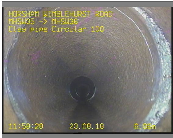
Photo: 35_35_217_A.JPG 6.06m, Crack, circumferential at joint, from 11 to 3 o'clock
