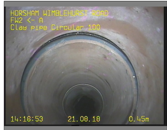
Photo: 13_13_61_A.JPG 0.45m, Joint displaced, medium
