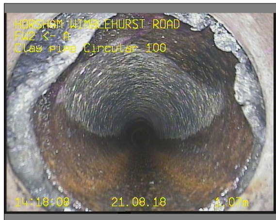
Photo: 13_13_62_A.JPG 1.07m, General remark Remarks: CONCRETE AROUND JOINT
