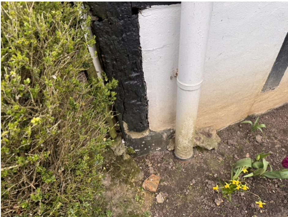
Photo (xii) – decayed bottom section of corner post with cement mortar repair
