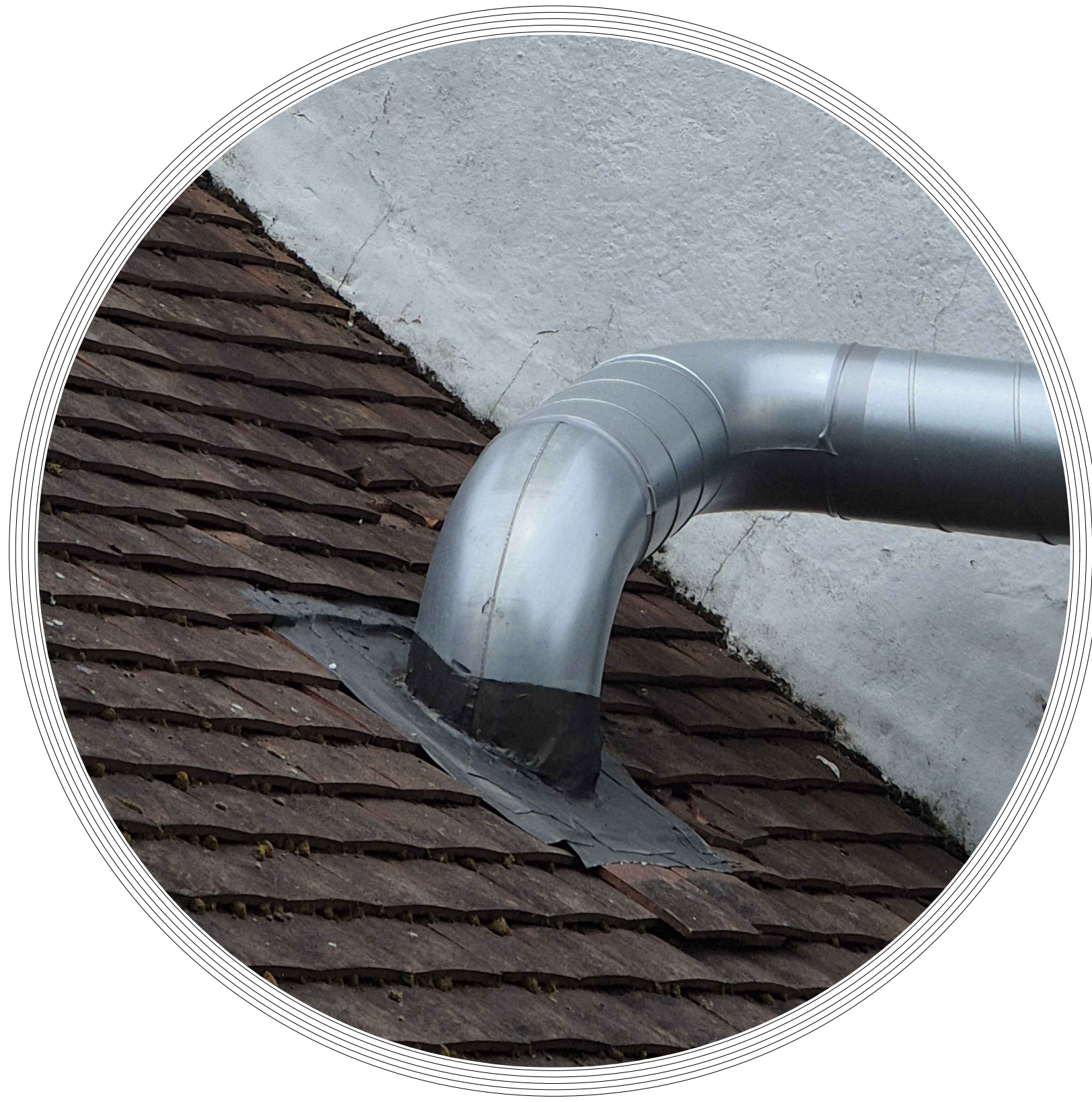
Extract Roof Junction dated 31.05.2026
