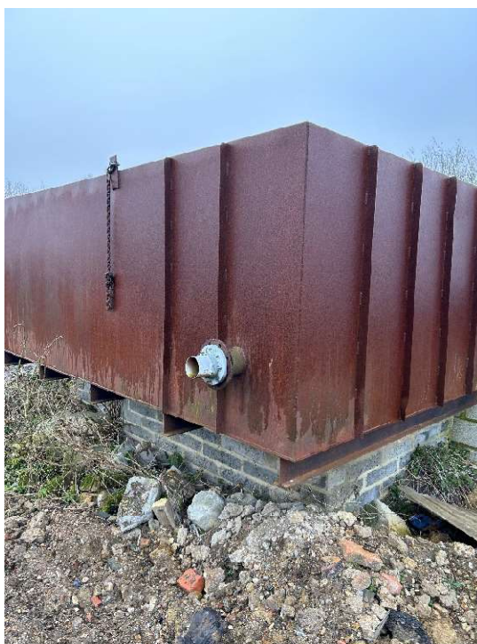
Photo 8: Redundant tank adjacent to pigstie.
