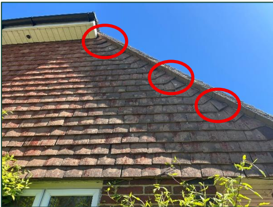
B1: Gaps under tiles on the southern elevation
