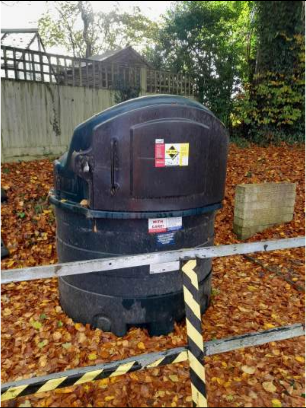
Plate 20 – Oil storage in the south east corner of site looking south
