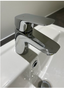
bathroom tap to basin
