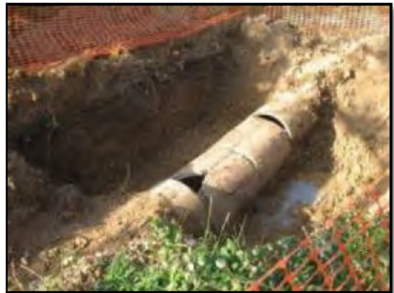
A damaged culvert requiring repair
