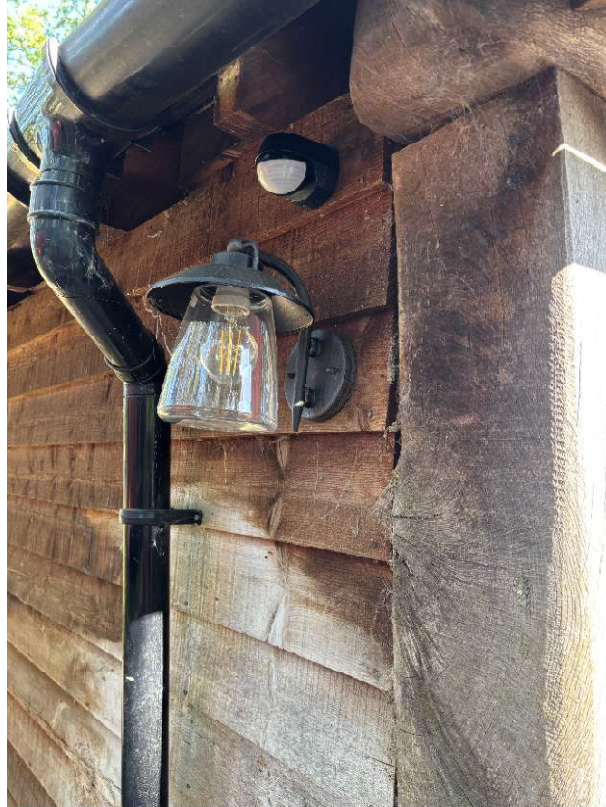
Garage light with PIR
