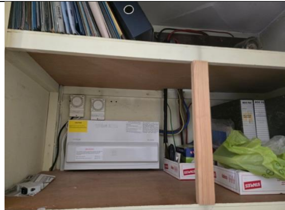
No 70 modern electrics, room F.01 (office)
