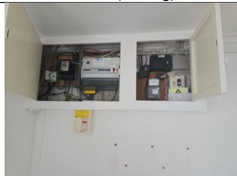
No 68 Modern electrics room G.01
