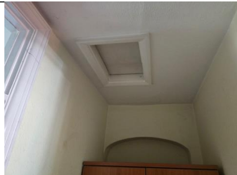
No 70 room F.02 (no access to loft, hatch too small)
