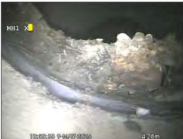
Photo: 35_7a, 00:00:00 5.1m, Debris silt, 25 % cross-sectional area loss
