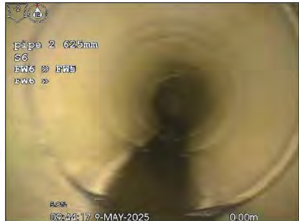
Photo: 2_5a, 00:00:00 0.4m, Joint displaced. Medium
