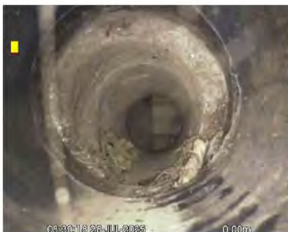
1, 00:00:04, 0.12 m Roots, fine at joint
