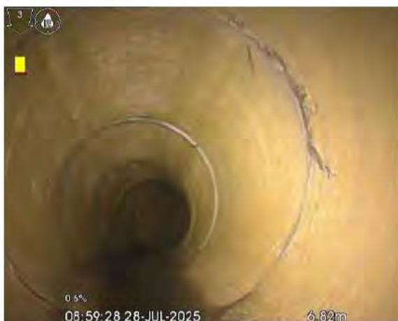
3, 00:00:44, 7.38 m Roots, fine at joint
