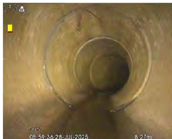
4, 00:00:54, 9.22 m Roots, fine at joint
