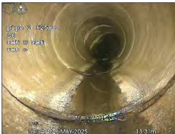
Photo: 26_12a, 00:00:00 13.6m, Joint displaced. Medium
