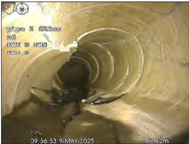
Photo: 28_13b, 00:00:00 17.25m, Circumferential Crack, from 06 to 11 o'clock
