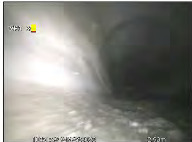
Photo: 33_5a, 00:00:00 3m, Debris silt, 10 % cross-sectional area loss
