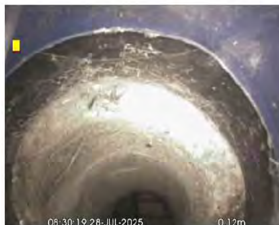
2, 00:00:04, 0.14 m Open joint, large
