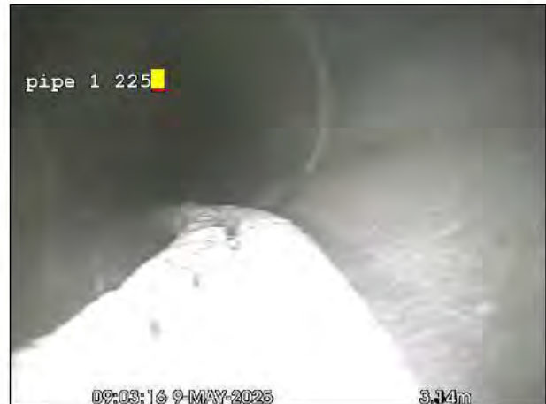
Photo: 4_4a, 00:00:00 3.2m, Obstruction, 15 % height/diameter loss
