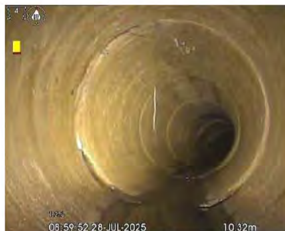
6, 00:01:13, 11.16 m Roots, fine at joint
