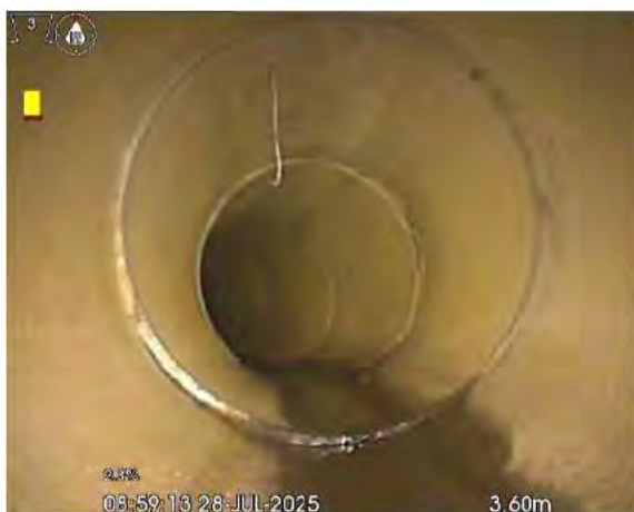
1, 00:00:30, 4.60 m Roots, fine at joint
