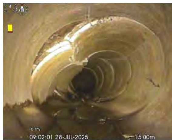
8, 00:01:49, 15.00 m Broken pipe from 12 o'clock to 12 o'clock, start
