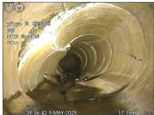
Photo: 28_13a, 00:00:00 17.25m, Circumferential Crack, from 06 to 11 o'clock
