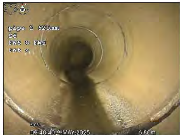
Photo: 2_8a, 00:00:00 7.1m, Joint displaced. Medium
