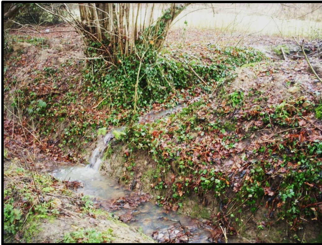
Photo 13: A drainage ditch from the field discharging into the ditch alongside Hollands Lane
