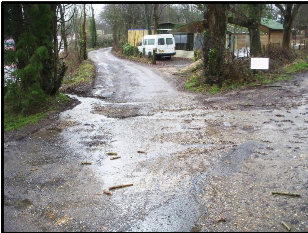
Photo 16: The junction of Hollands Lane (right) with the Rye Farm track (ahead) showing how runoff from the field damages the surface.
