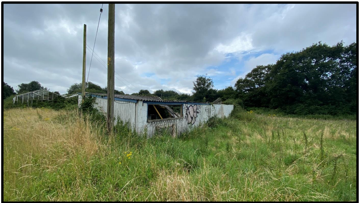
Photo 4: The ruined garage/workshop building looking south-west. An overhead cable once brought electric power to the building.
